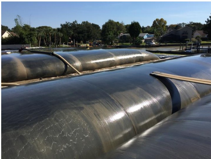
The Triflo Mechanical Dewatering System separates the sediments, while fine mesh filters remove and clean the water, which is returned to the canal.
